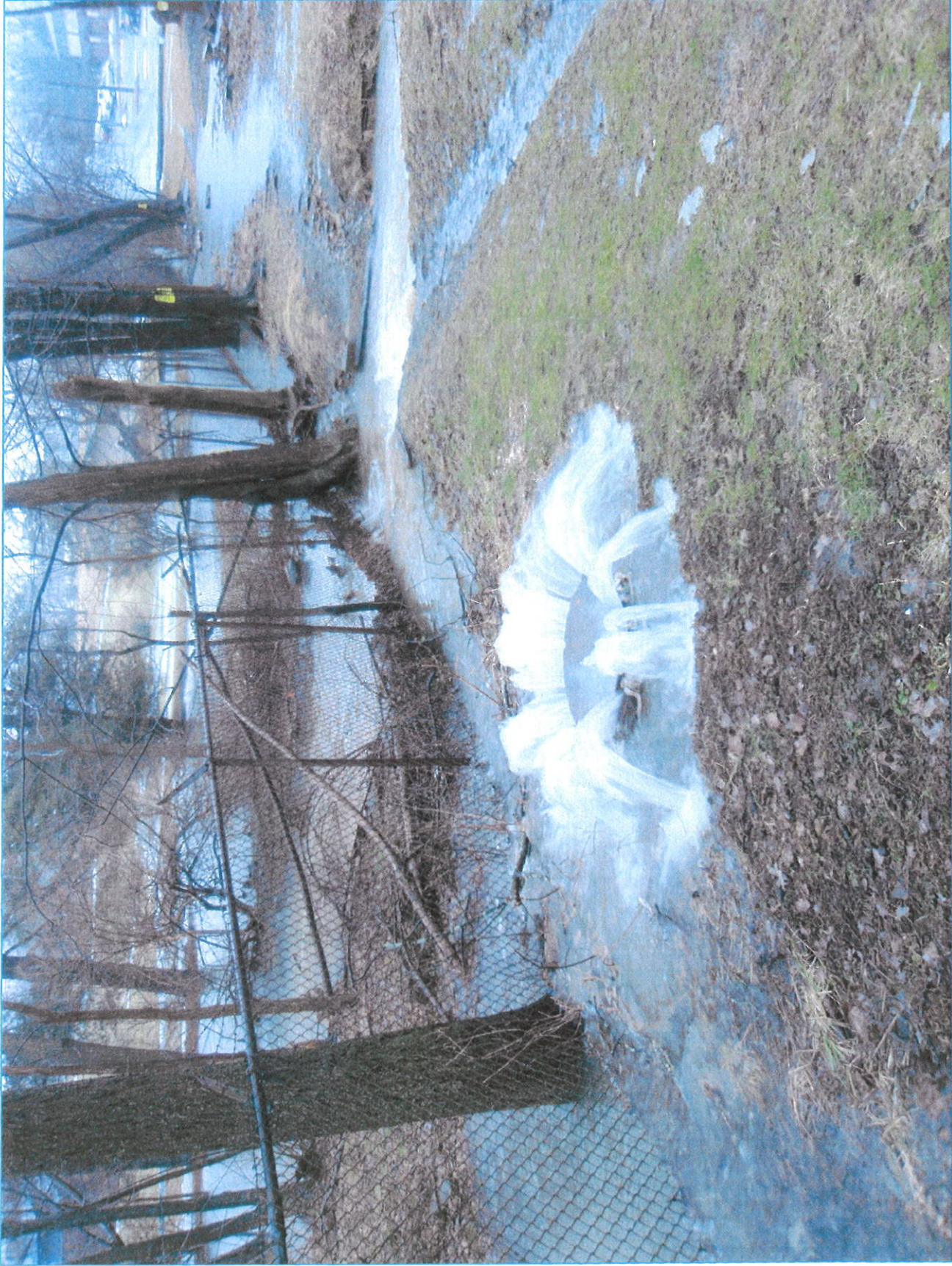
OVERFLOWING MANHOLE - MARCH 8, 2008 CANTRELL AVENUE, NEAR CLEMSON PARK CONDOMINIUMS SEWER SLOPE UPSTREAM AND DOWNSTREAM IS FLAT-TO-GENTLE
